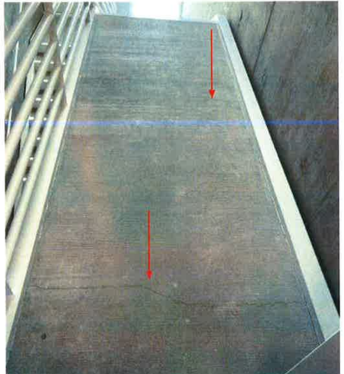
#19. Upper level landing Stair S-2, floor cracking.
