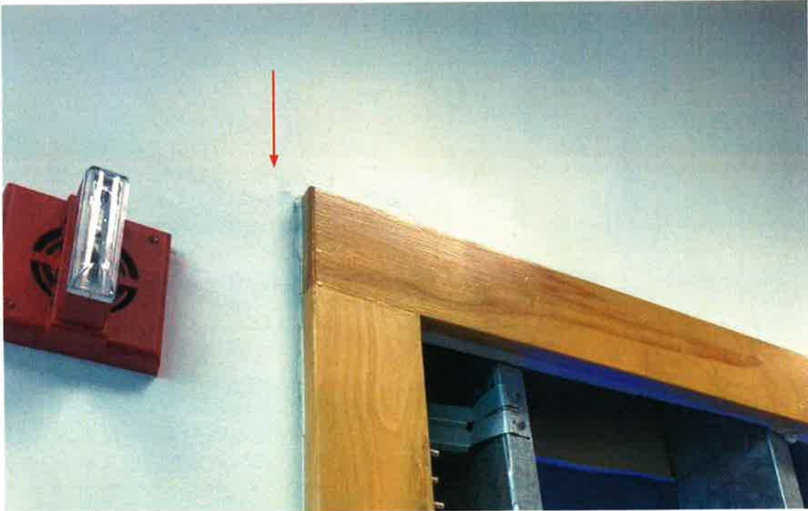
#7. Gypsum board movement observed at millwork corner
