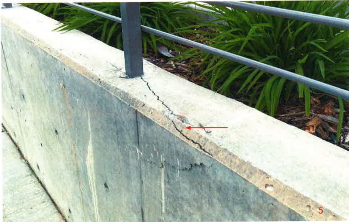
#3 Retaining concrete wall cracks
