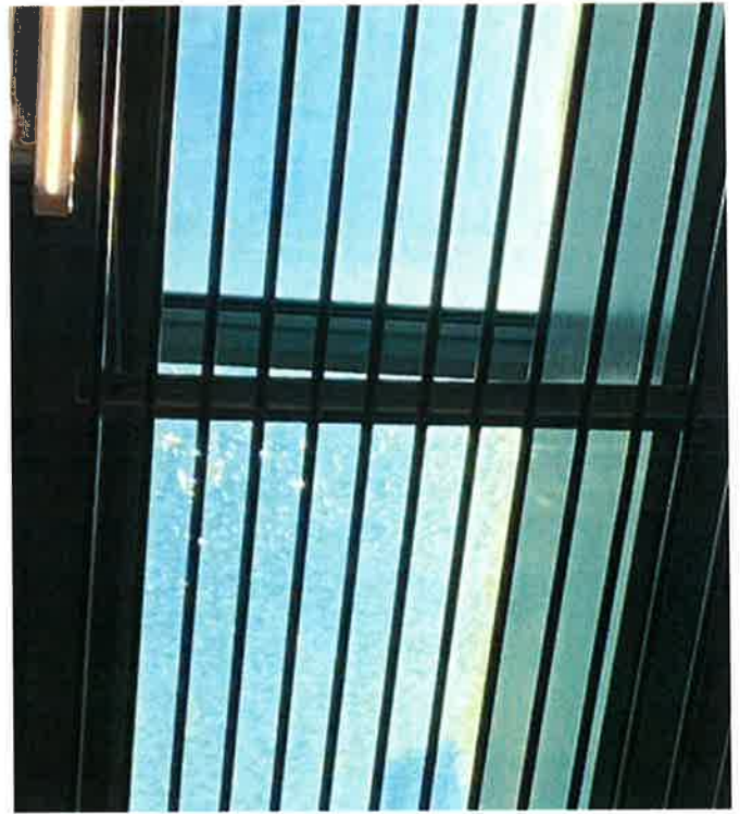
#8. Shattered glass at skylight. View from roof and stacks area.
