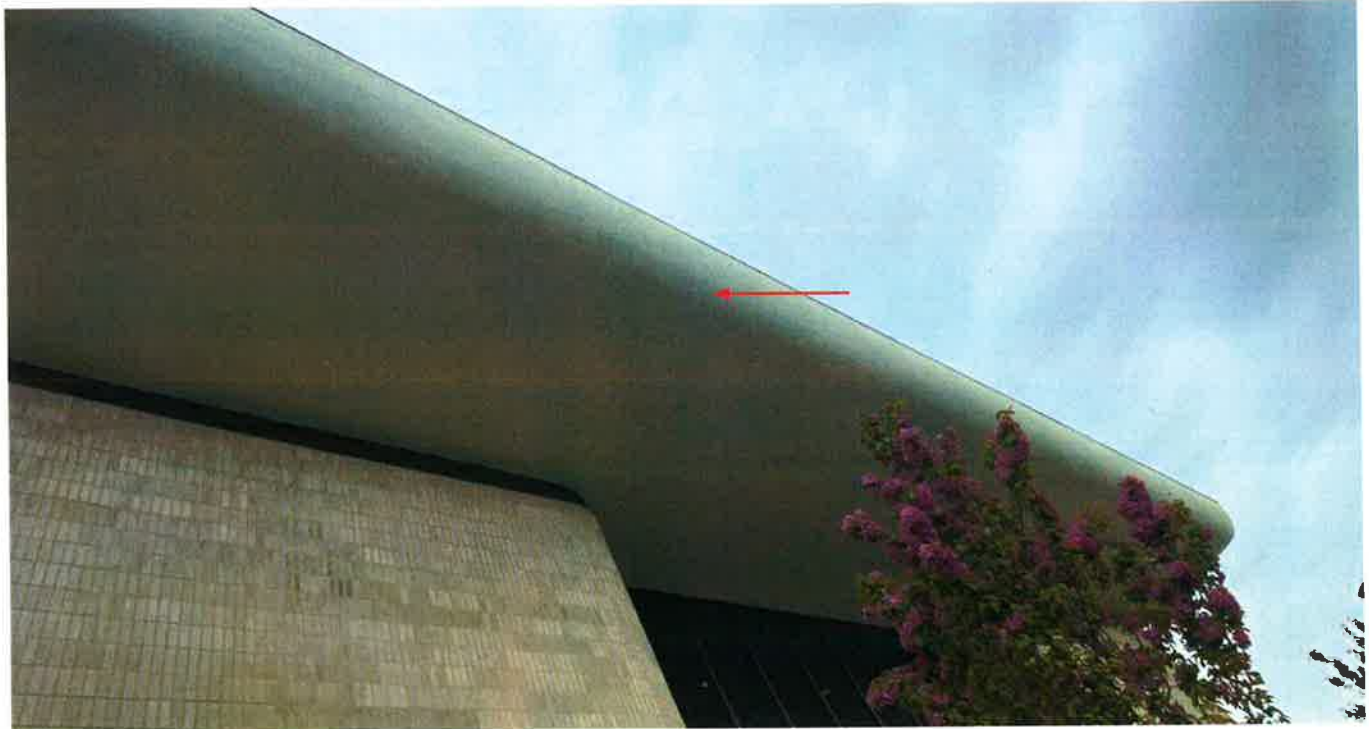
#1. Plaster Soffit hairline cracks
