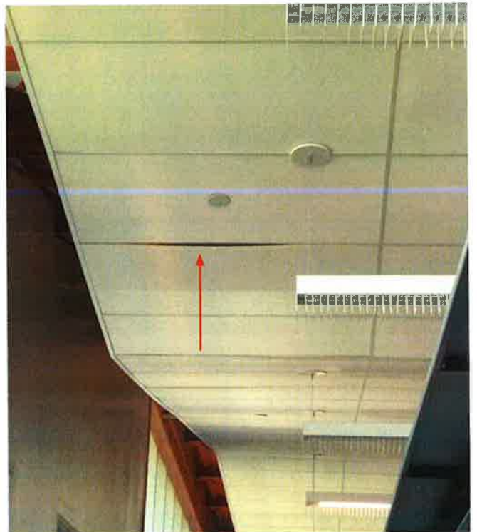
#9. Acoustical ceiling panel displaced from grid
