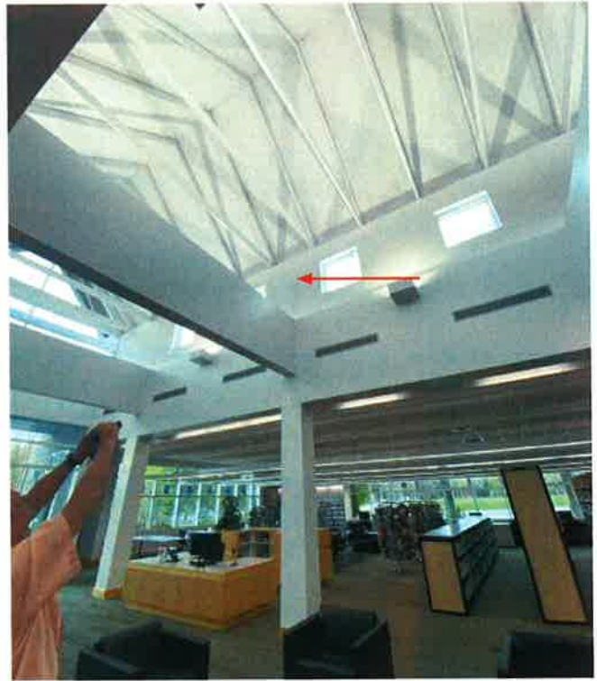
#5. At central skylight, gypsum wall cracking was observed
