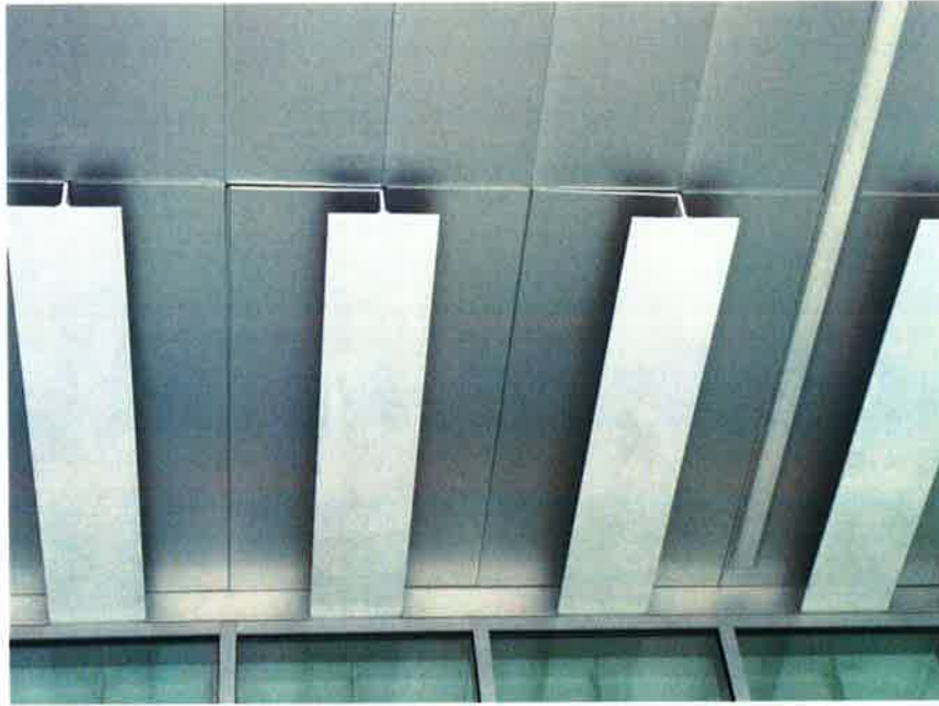
Photo #5 – Exterior soffits appear to have shifted
