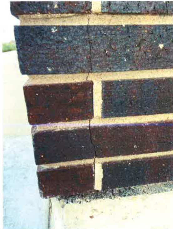
Photo 2 – Example of cracks propagating in masonry veneer
