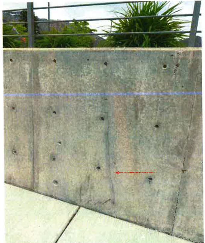
#3 Retaining concrete wall cracks
