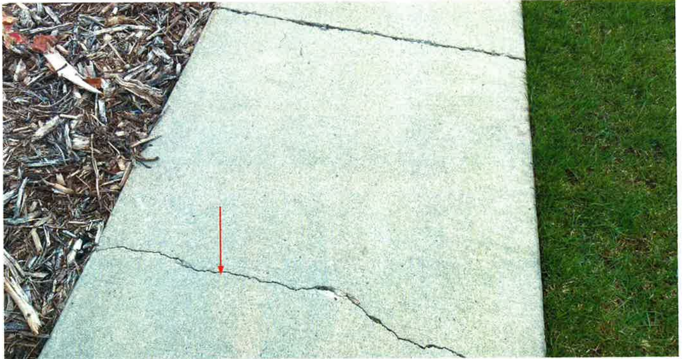
#2. Cracks at entrance walkway concrete slab on grade
