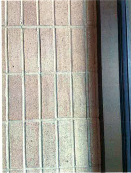
Photo #3 – Example of cracks brick veneer
