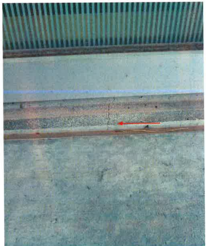
#6. Hairline crack at foundation wall at South Glazing.
