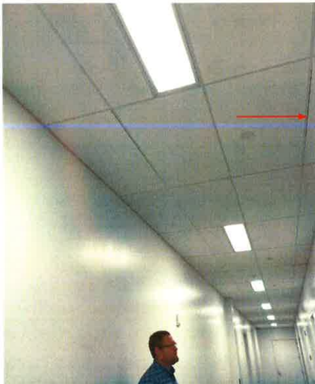
Maintenance Area SR Hall cracks at ceiling tile movement
