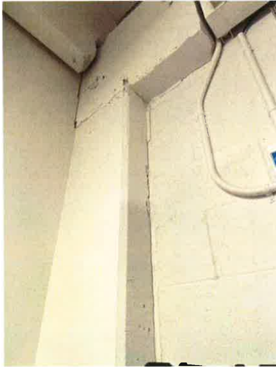
Photo #5 – Example of cracks in masonry and concrete walls
