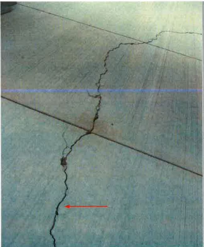
#1.Exterior plaza cracking
