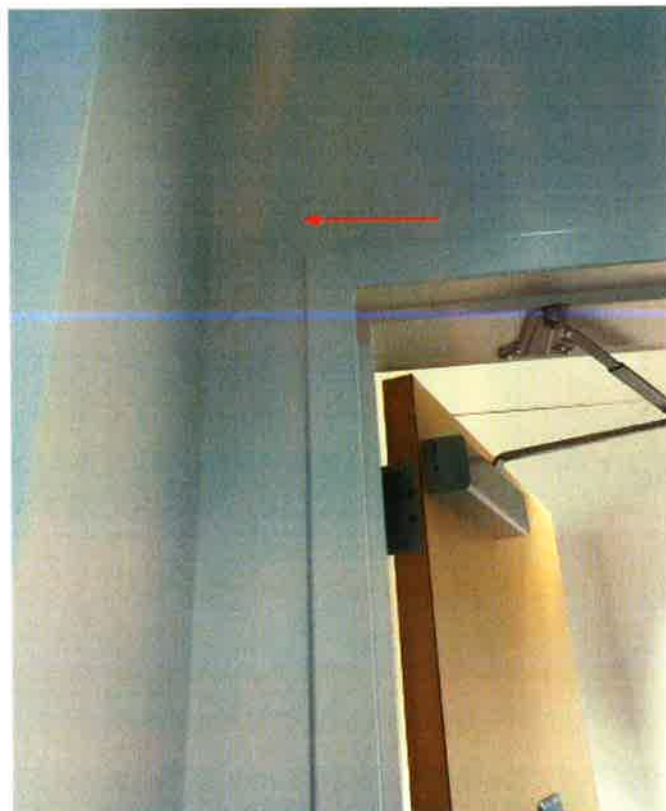
#3. Gypsum board wall cracks at door frames
