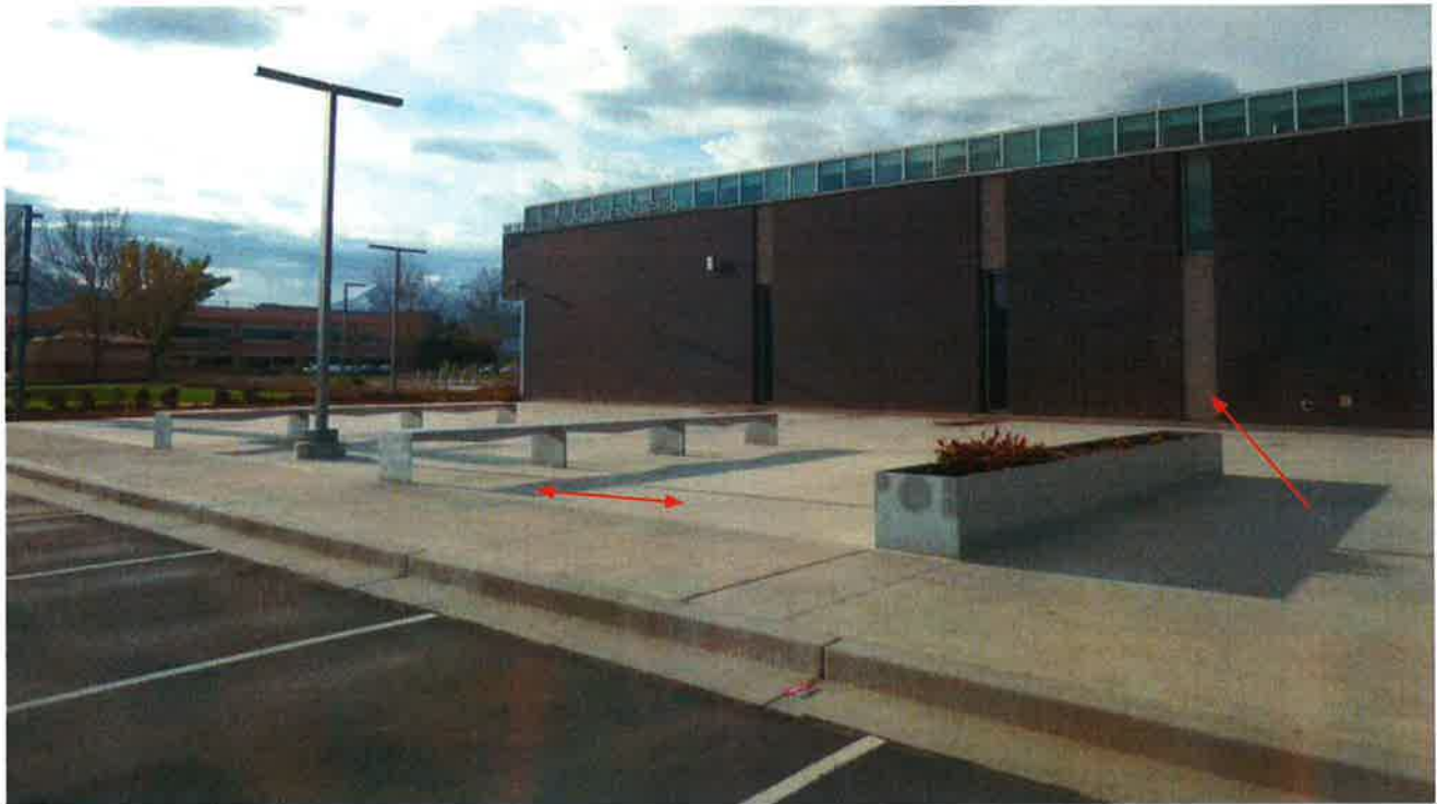
North Facade plaza and typical brick masonry reliefs where damage was observed
