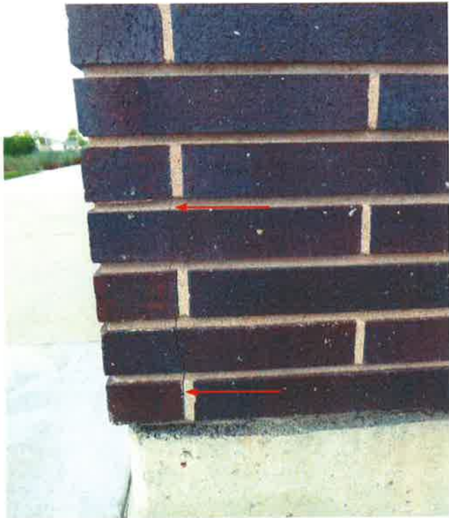
#5. Brick masonry damage.
