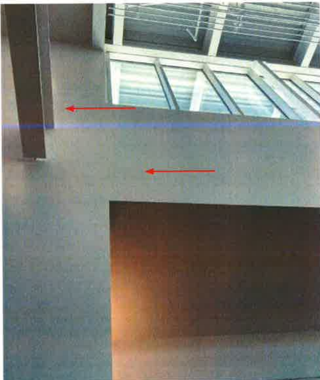
#10 and #11. Painted Gypsum Board wall crack
