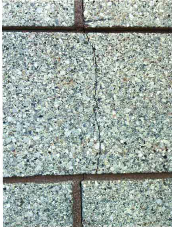
Photo1 – Example of cracks propagating in masonry wall
