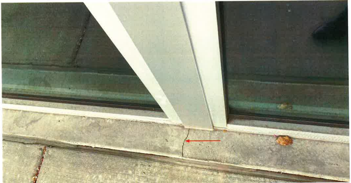
#2. Lower level South entrance foundation wall cracks
