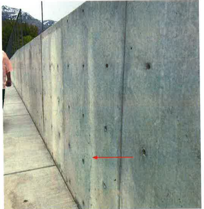
#3 Retaining concrete wall cracks
