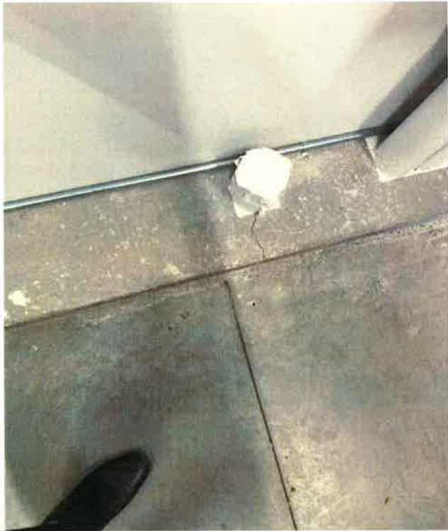
#18. Maintenance Area SR Hall cracks at concrete floor.
