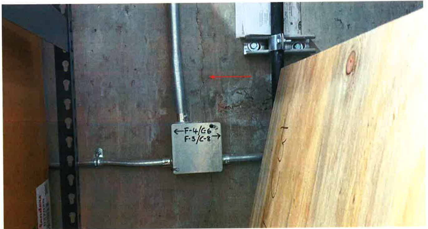
#5. Lower level storage room exhibits cracks at concrete structure
