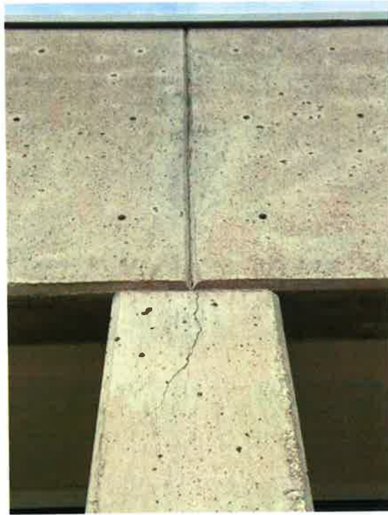
Photo1 – Example of cracks in exterior beams and columns
