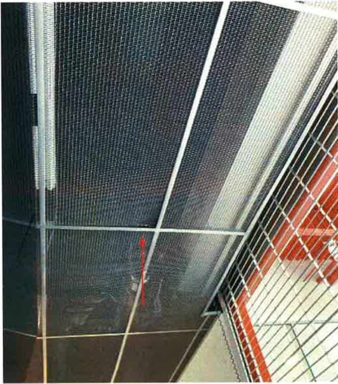
#9. Acoustical ceiling panel displaced from grid
