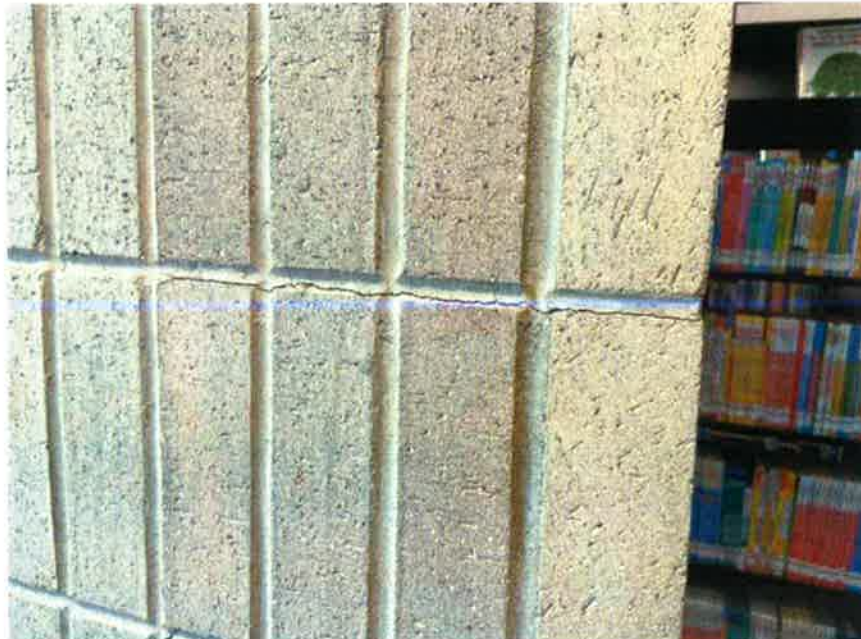
Photo 2 – Example of cracks in brick veneer
