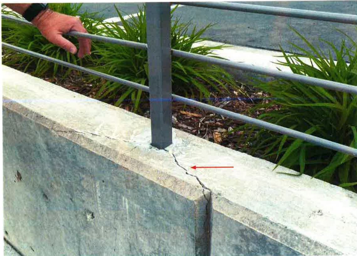
#3 Retaining concrete wall cracks
