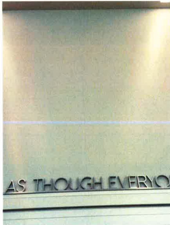
Photo #8 – Example of a crack in the sheetrock wall
