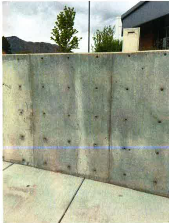
Photo #4 – Example of cracks in retaining wall
