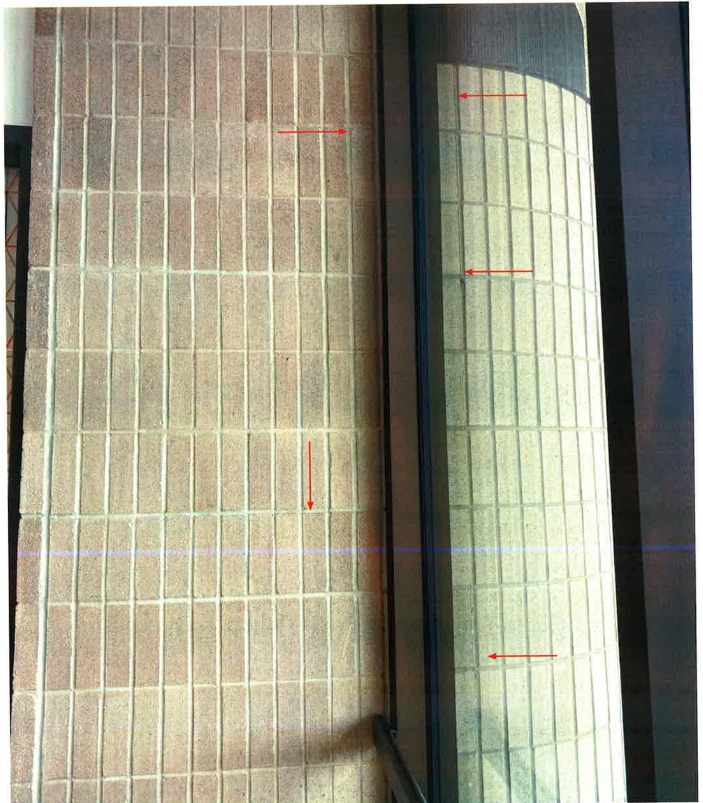
#2. Brick masonry joint cracking
