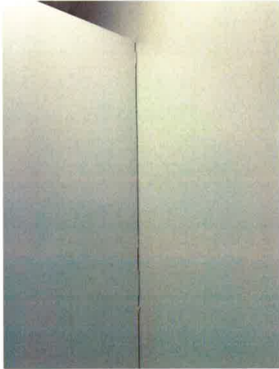
Photo #7 – Example of cabinet pulling away from wall
