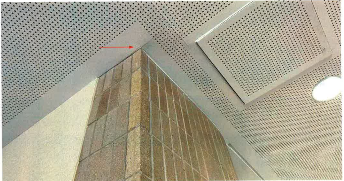
#7. Ceiling separation from wall
