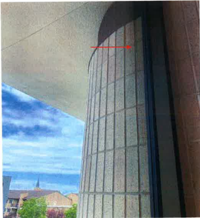
#2. Brick masonry joint cracking on level 2
