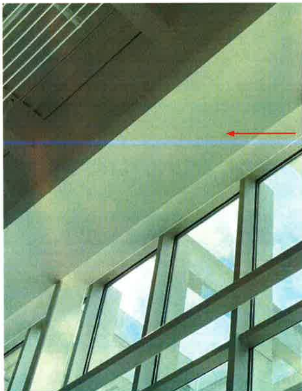
#16. Ceiling above South glazing cracks.
