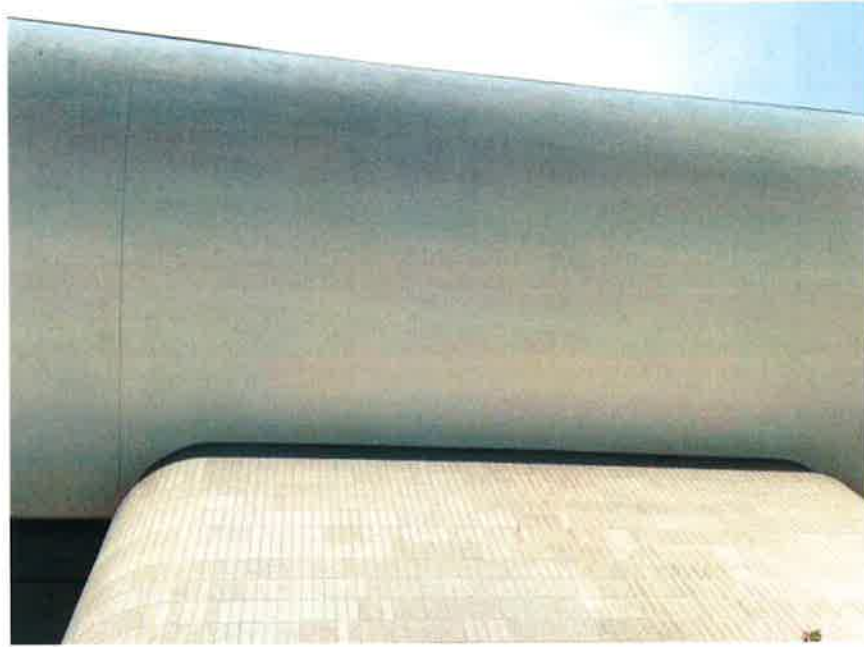
Photo #5 – Example of cracks in exterior soffit
