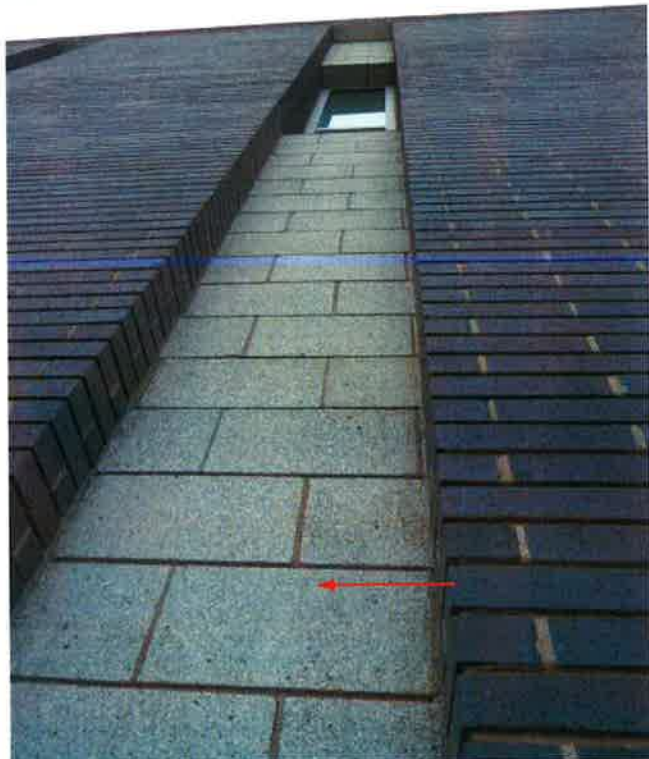
#2. North and East masonry wall cracking.
