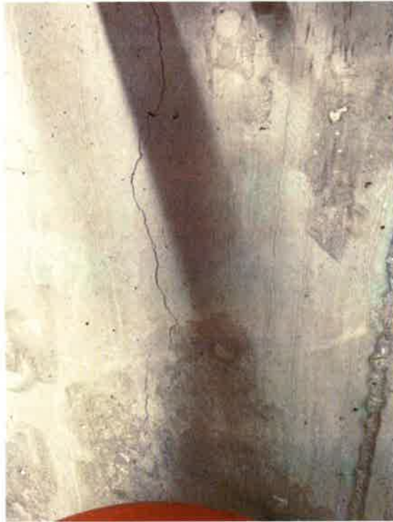
Photo1 – Example of cracks in foundation walls
