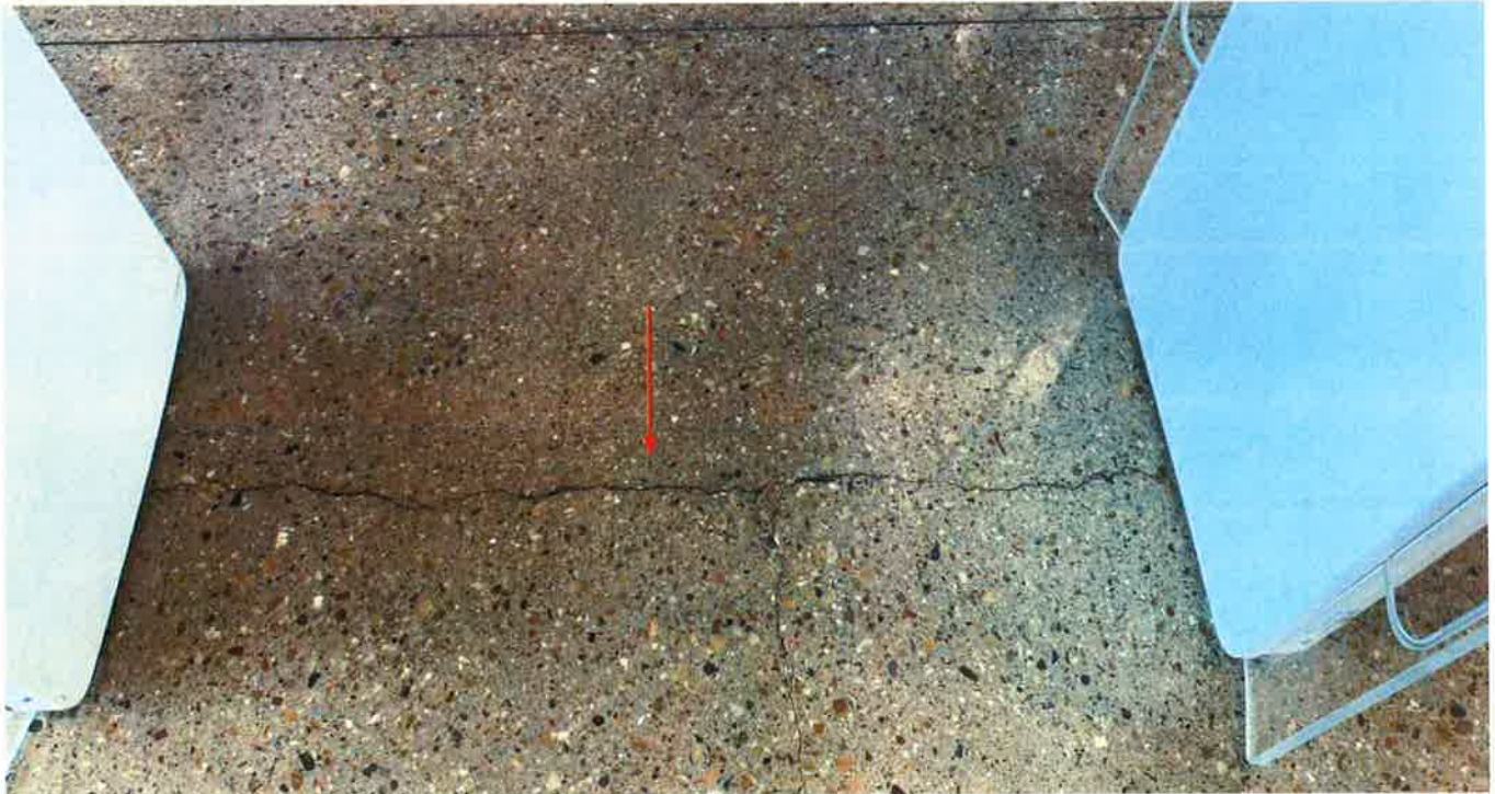
#6. Concrete floor cracks at public circulation areas
