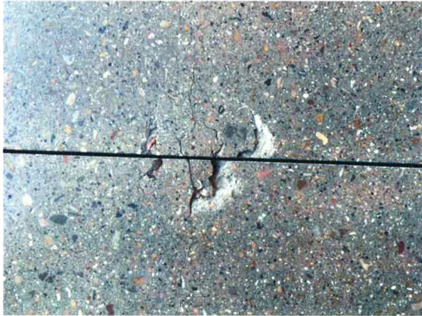
Photo #3 – Example of cracks propagating in slab on grade
