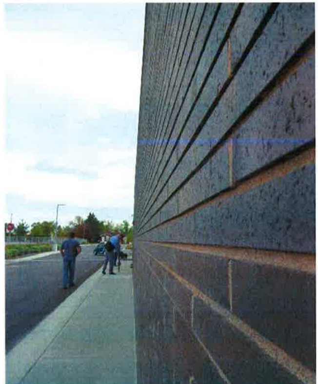
In general, brick masonry appears leveled and without out of plan movement
