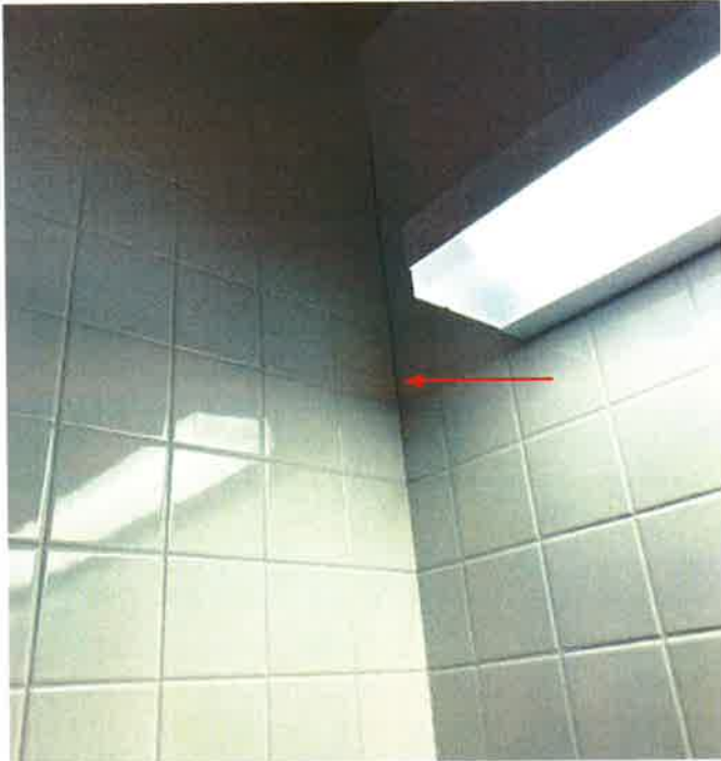
Ceramic tile joints movement at walls intersection
