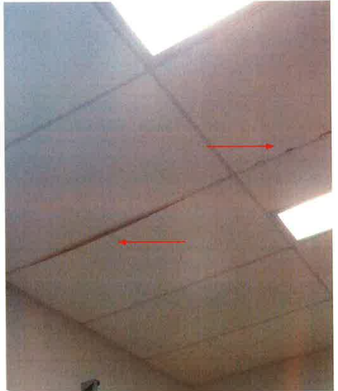
#13. Kitchen ceiling tiles surface cracking and shifting from ceiling grid
