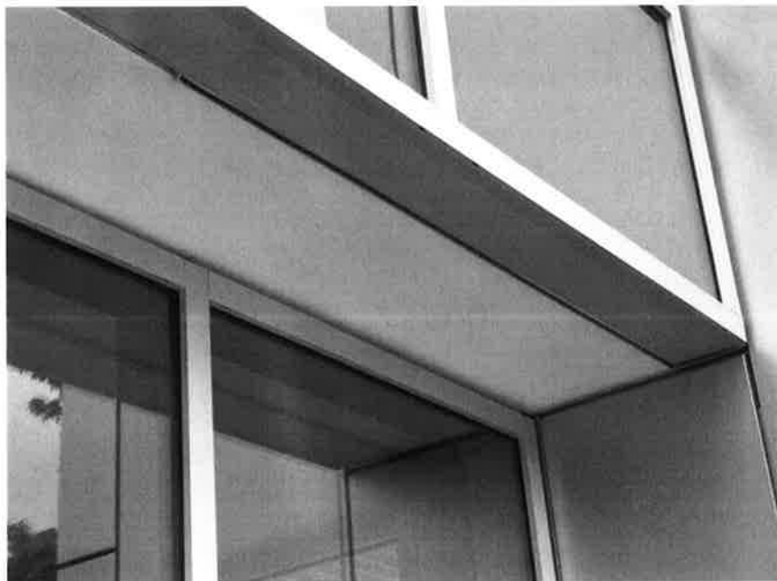
Photo 2 – Example of exterior soffit panel out of place
