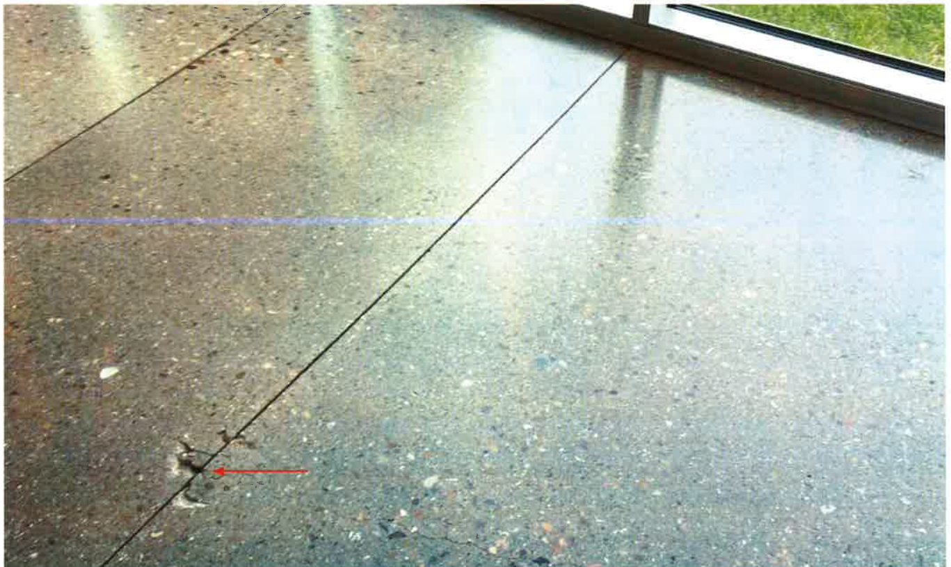
#6. Concrete floor cracks
