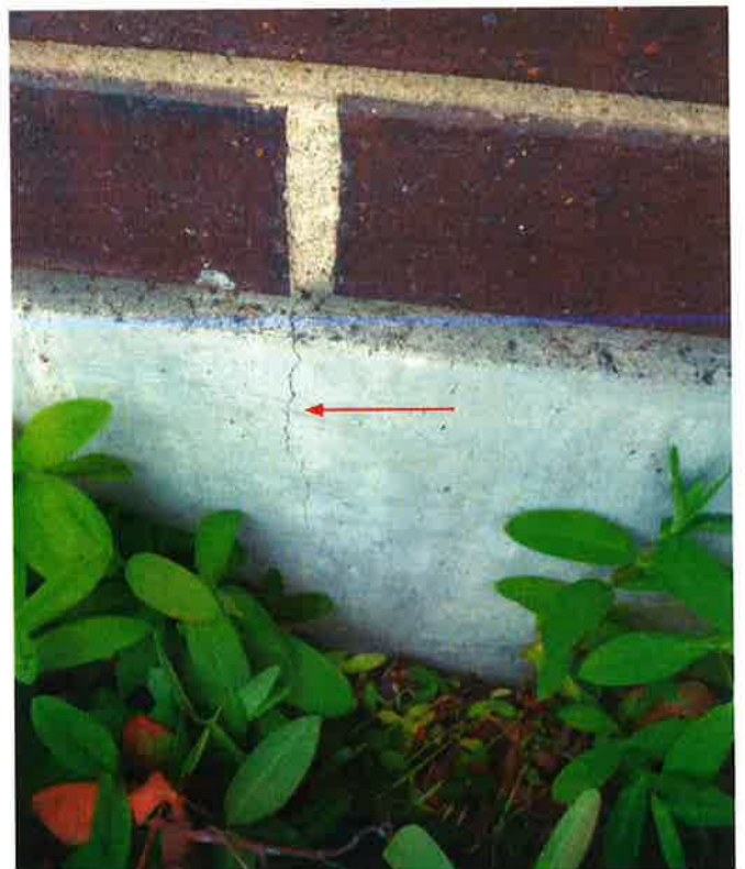
#3. North and East foundation wall cracking.
