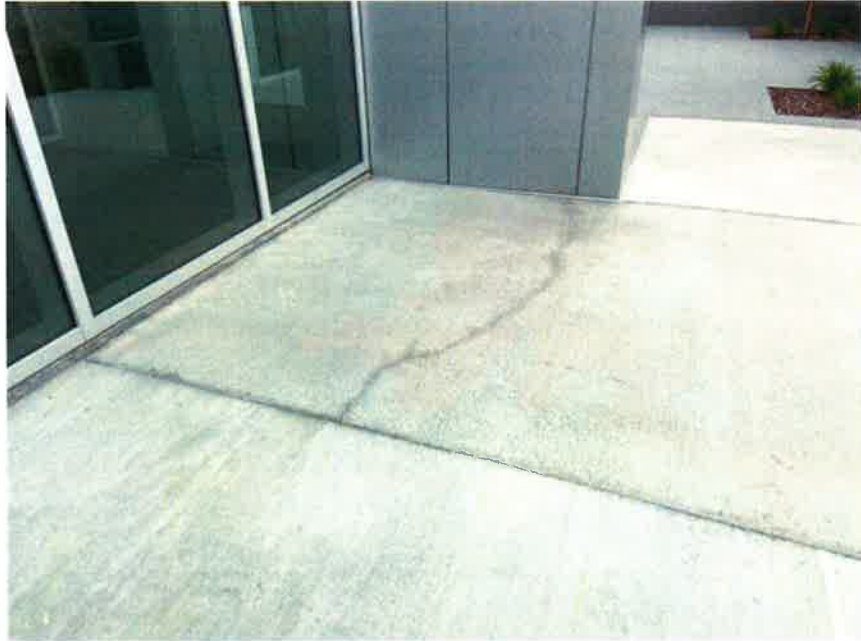
Photo #3 – Example of cracks in slab on grade
