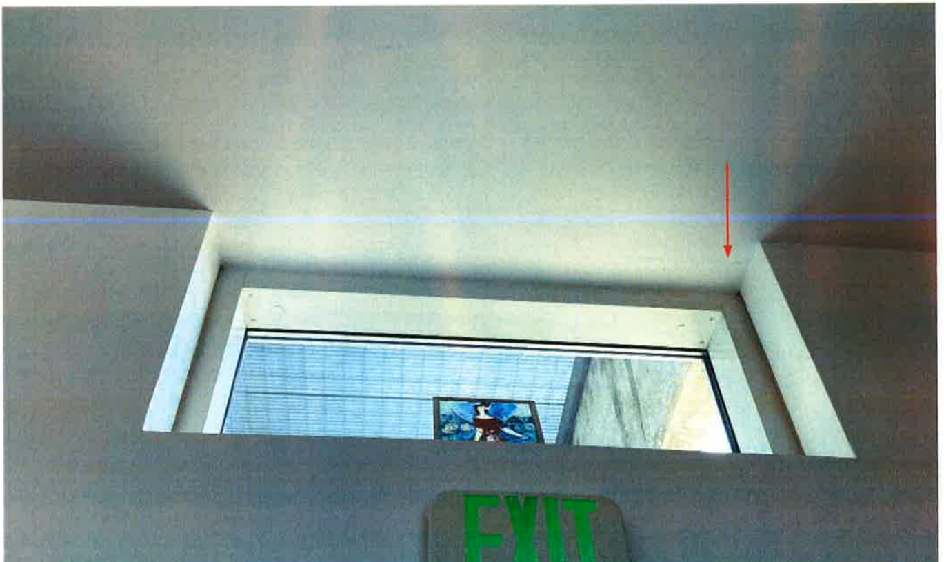
#7. Hairline crack at painted gypsum wall surface
