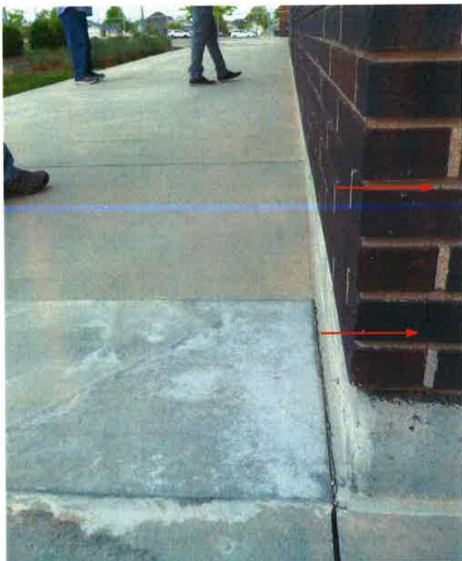
#5. Brick masonry damage.
