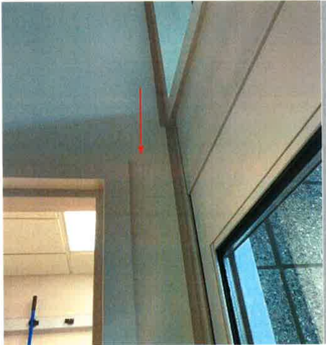
#3. Gypsum board wall cracks at door frames
