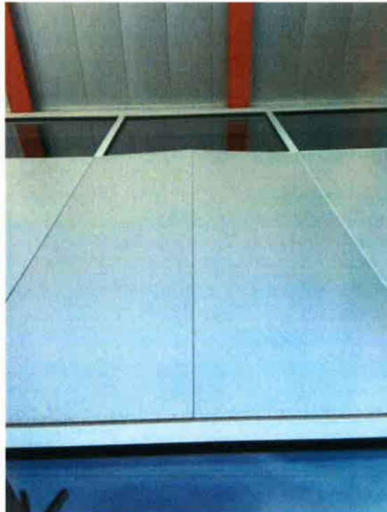
Photo 2 – Example of exterior panel buckling out-of-plane
