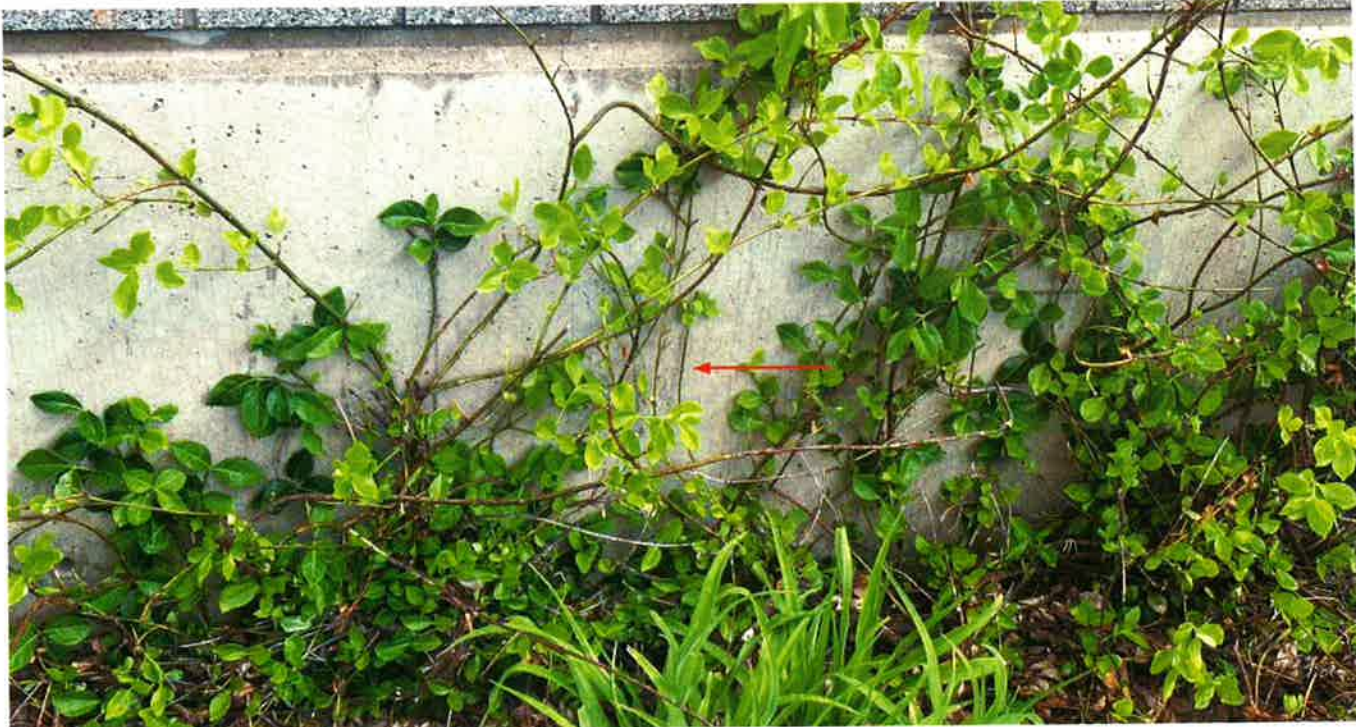
#1. Concrete walls hairline cracks
