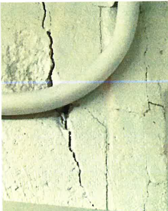
#5. Lower level storage room exhibits cracks at concrete structure
