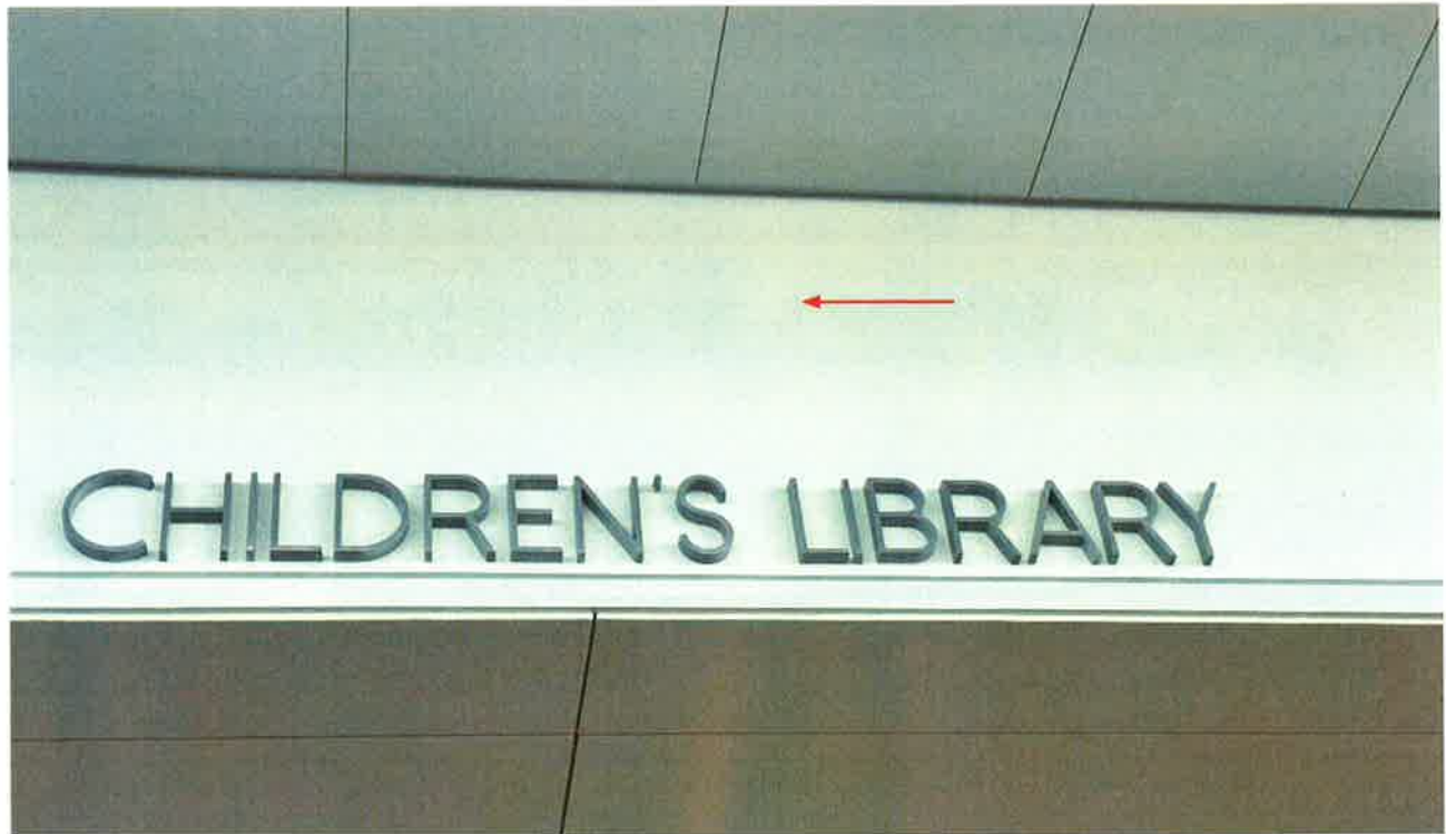
15. Children's Area, Gypsum Board crack
