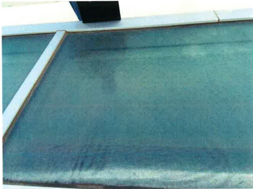
Photo #8 – Broken window in skylight
