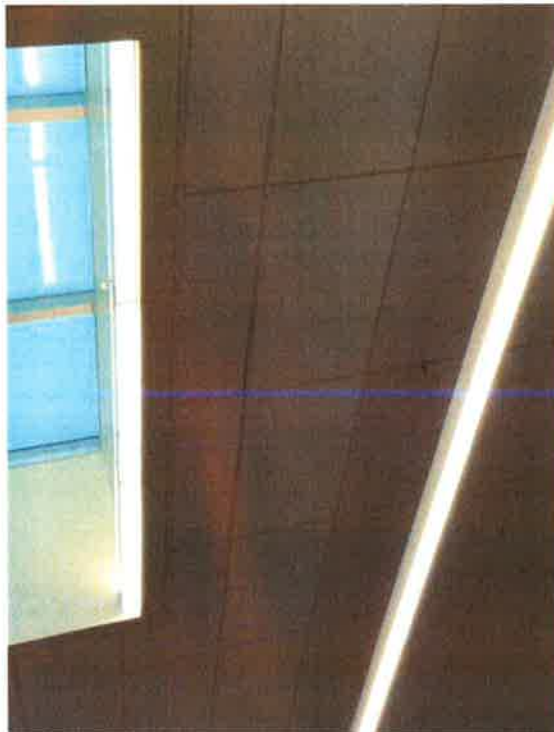
Photo #6 – Example of displaced ceiling tile
