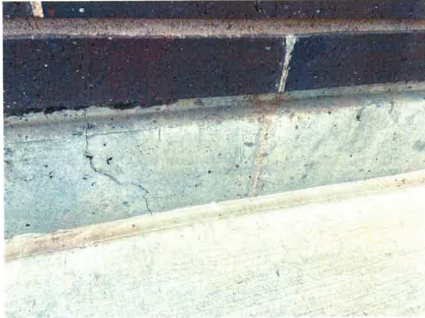
Photo #3 – Example of cracks propagating in foundation wall
