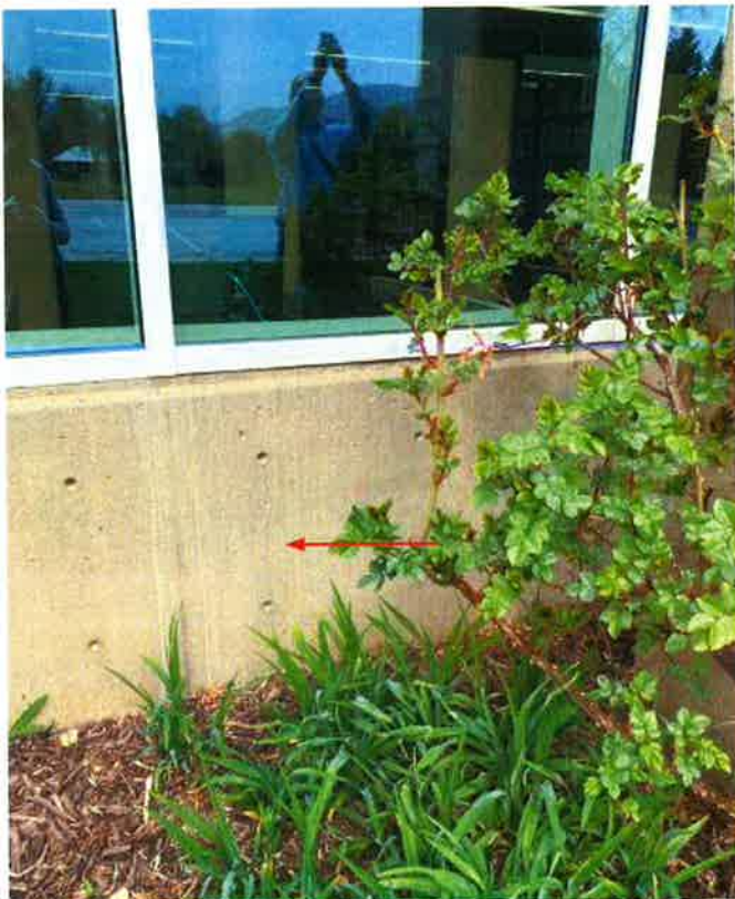
#1. West exterior wall hairline cracks at concrete wall
