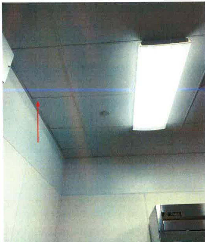
#9. Acoustical ceiling panel displaced from grid
