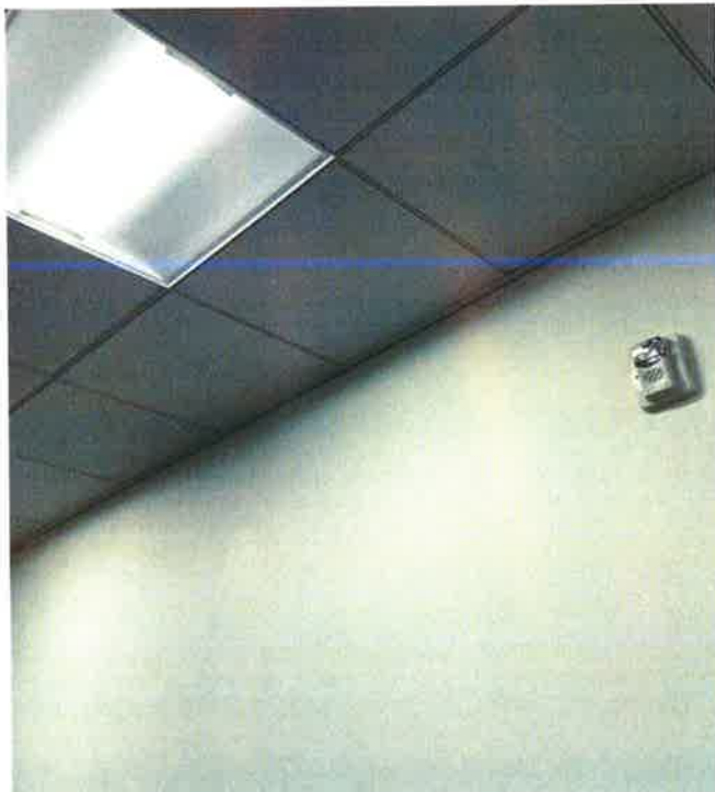
#6. Ceiling tile displacement
